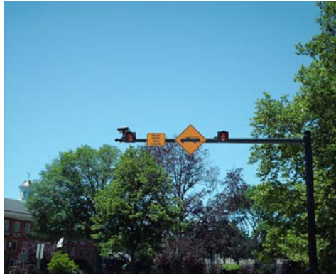
Figure 1: Horizontal Mast Mounted Warning Beacon
